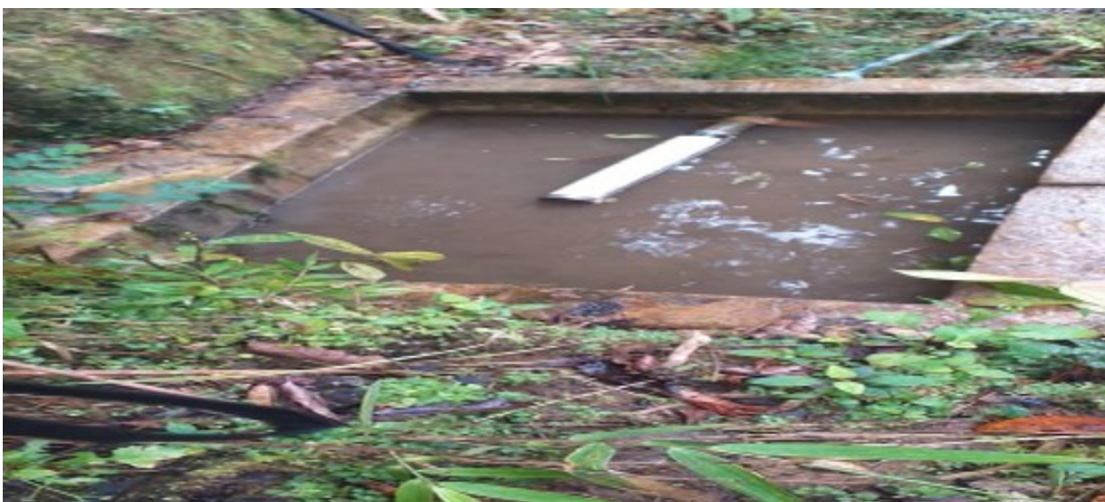
Photo of Sump that needs to be capped to finish Komea PNG Water project
