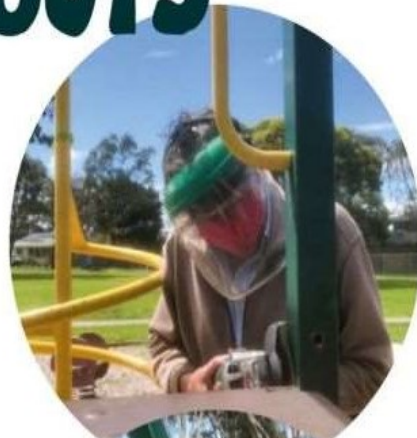
PICTURED (TOP TO BOTTOM): Terry Valentine takes a shortcut dismantling playground equipment after losing the battle with a stubborn bolt; Friend of Rotary Mel Bell coding the components of the playground so they can be reassembled correctly at the destination; The team discusses another stubborn bolt.
